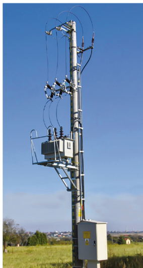
POLE MOUNT TRANSFORMER STATIONS
