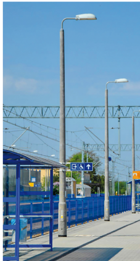
EOP TYPE LIGHTING RODS
