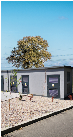
CONTAINER TRANSFORMER STATIONS
